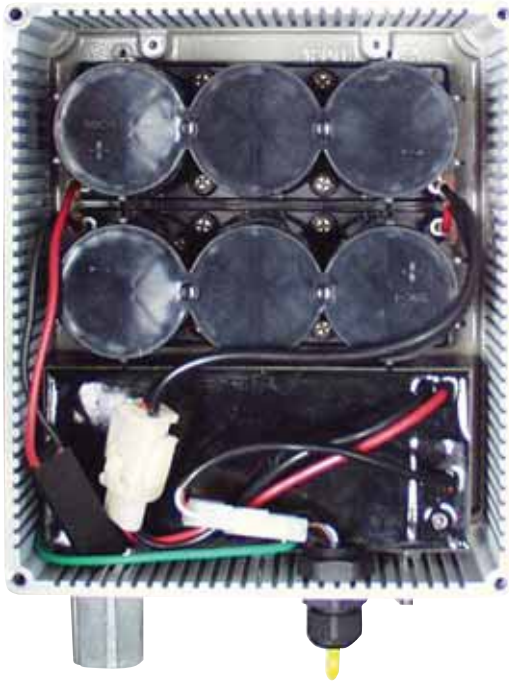
LPS AND BATTERY W/COVER REMOVED
